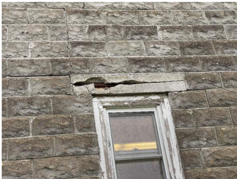
FAILING LINTEL AT SOUTH WALL
