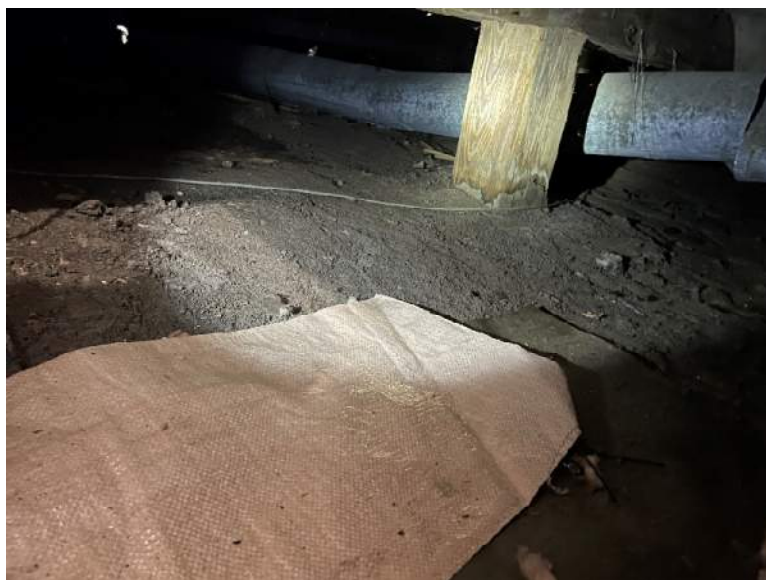
WATER STAINED POST IN CRAWLSPACE
