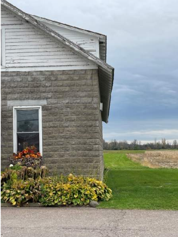
MASONRY CRACKING- NORTH AND WEST WALLS
