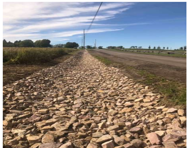
Figure 2.5: This new stone lined ditch on Kibbe Point Road was funded by Grants In Aid in 2022 and will reduce erosion and improve stormwater infiltration.
