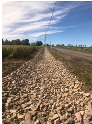
This new stone lined ditch on Kibbe Point Road was funded by Grants In Aid in 2022 and will reduce erosion and improve stormwater infiltration.
